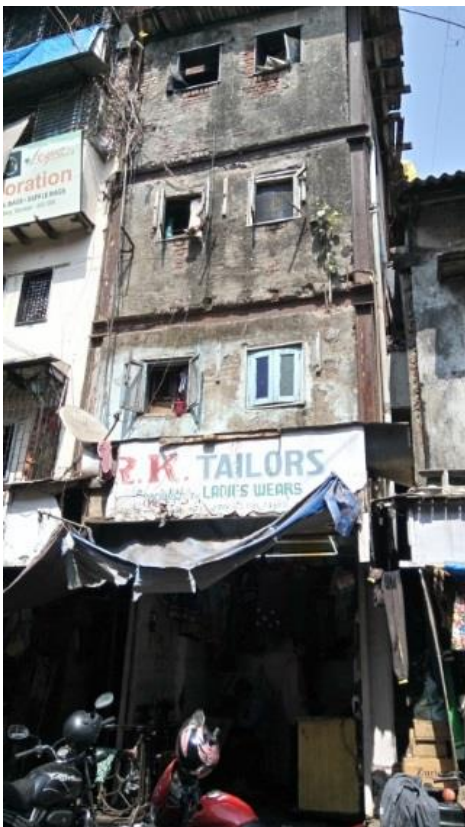
Figure 13 : Condition of Dilapidated Buildings
